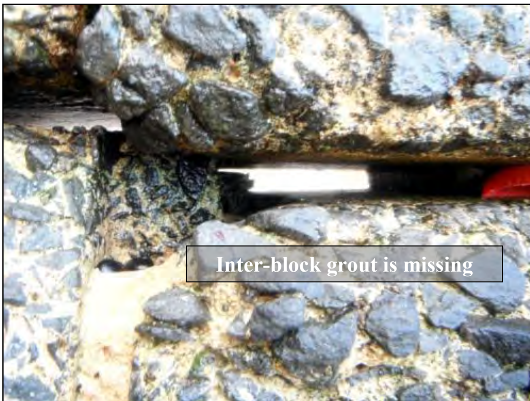
Figure 3-3 Looking between the blocks where the grout is missing.
