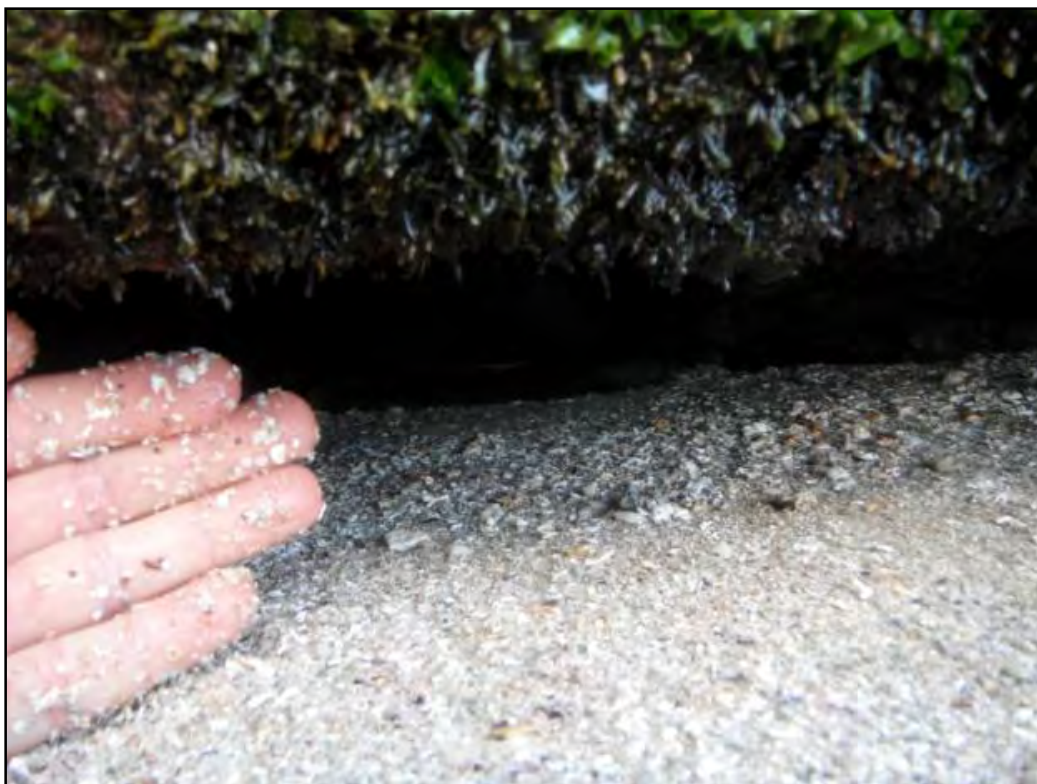
Figure 3-5 Gaps below base of structure are greater than four inches high in many locations.
