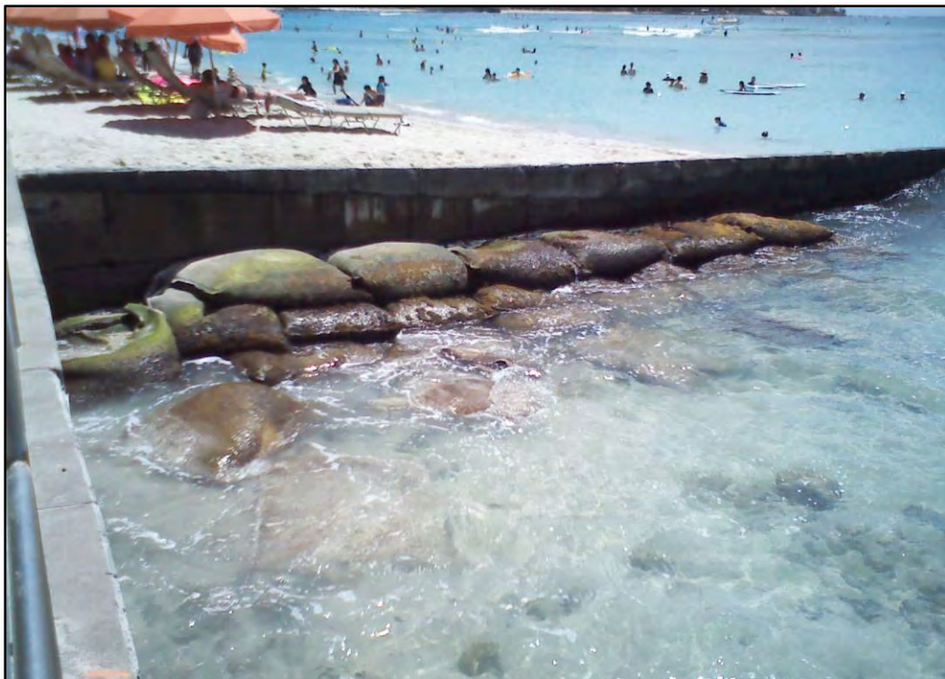
Figure 3-8 Several displaced ElcoRock sand bags (photo date September 24, 2014)
